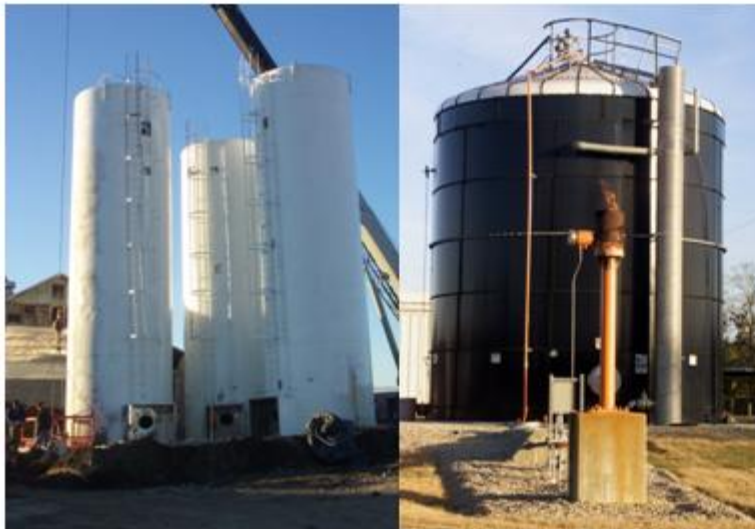
Anaerobic Sludge Blanket Attached Media
