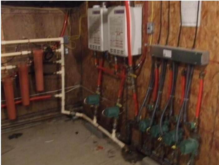
Tankless Hot Water Heaters & Circulation Pumps
