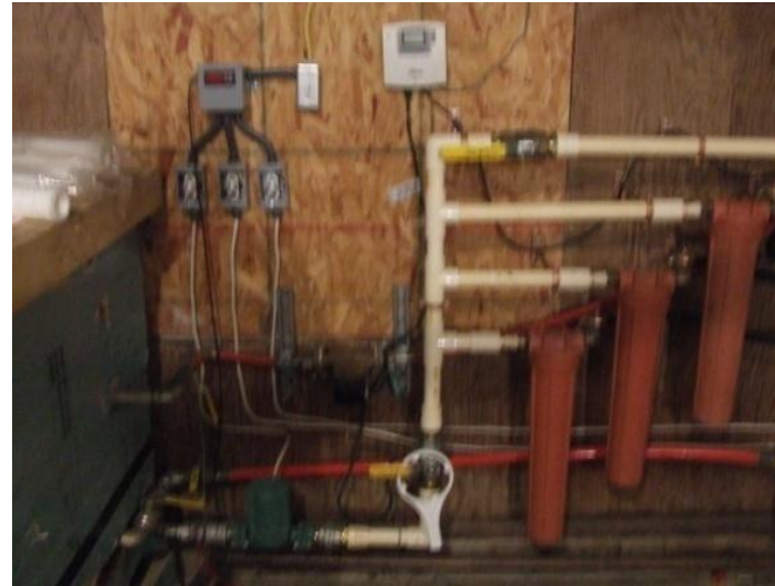
Controllers & Water Filtration (if applicable)
