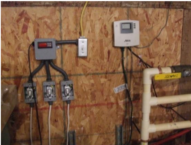
House, Water & Solar Temperature Controllers
