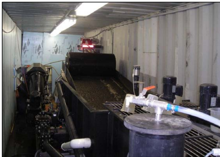
Figure 7. Interior of Kemira trailer, showing system
